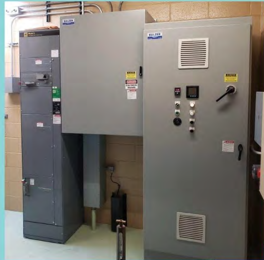
New motor control center
