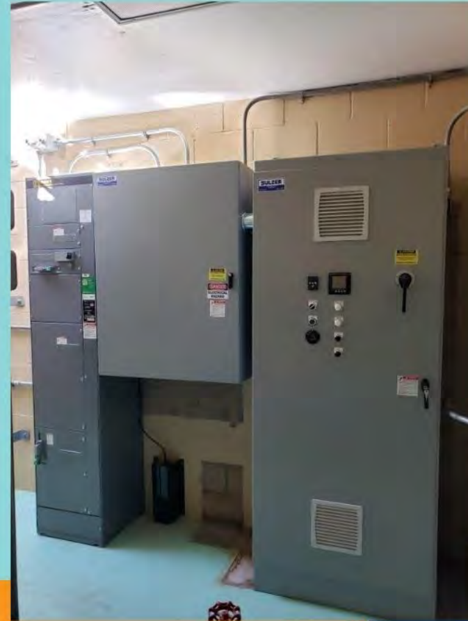
New motor control center
